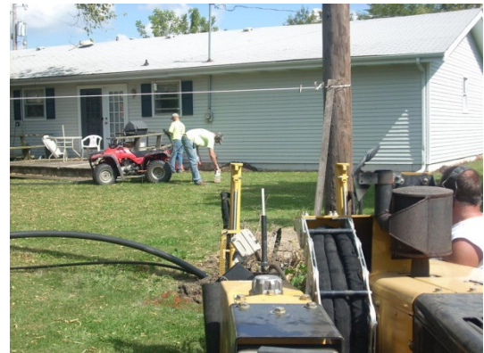
The City of Princeton is helping the environment while protecting its citizens. Putting overhead utility lines underground using HDPE conduit pipe reduces the need for the more than 800,000 wooden poles purchased by electric companies annually in the United States.
